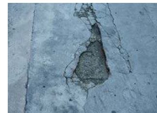
crevasses et fissures
